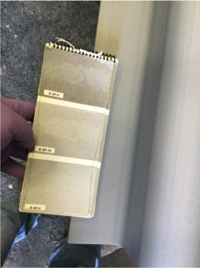
Photo Description: Grit blasted Surface visual comparison to SSPC -VIS 1 guide SP10 cleaning
