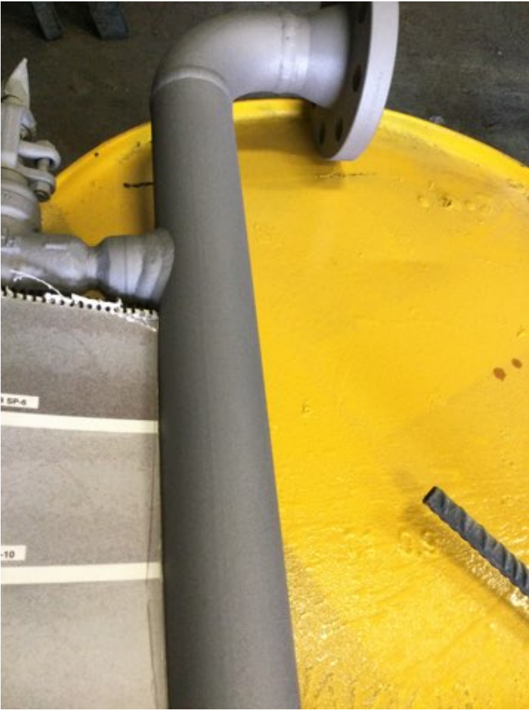
Photo Description: Grit blasted Surface visual comparison to SSPC -VIS 1 guide SP10 cleaning
