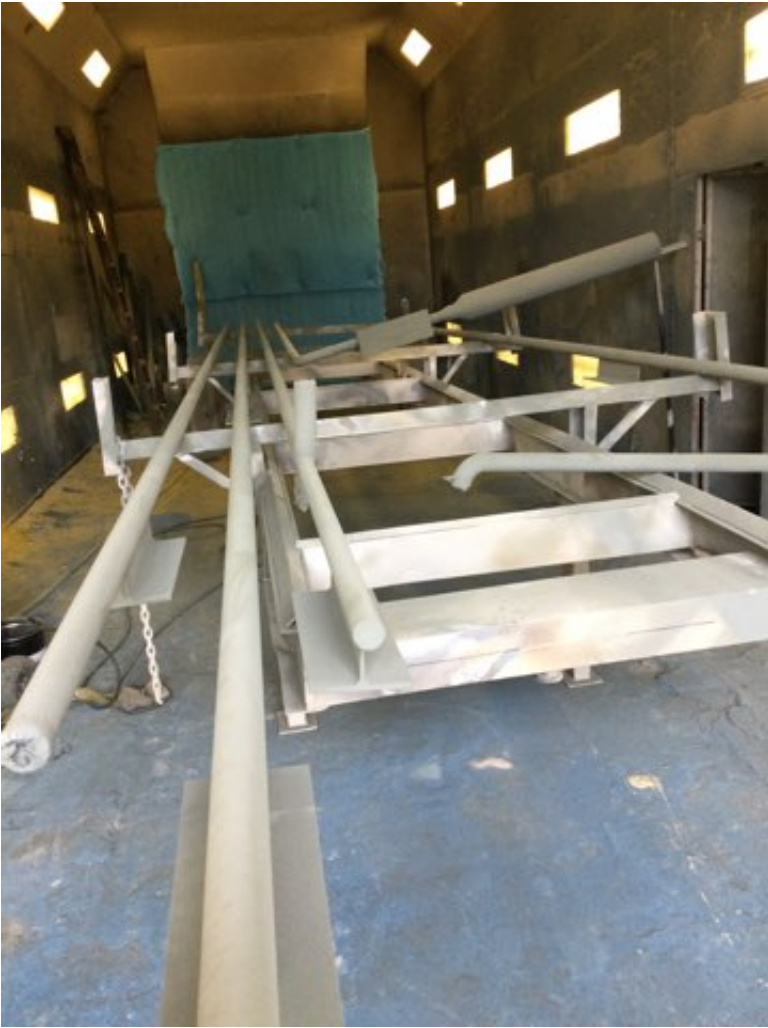
Photo Description: Zinc coating
