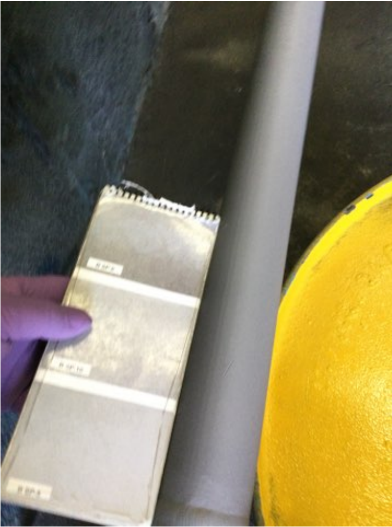
Photo Description: Grit blasted Surface visual comparison to SSPC -VIS 1 guide SP10 cleaning
