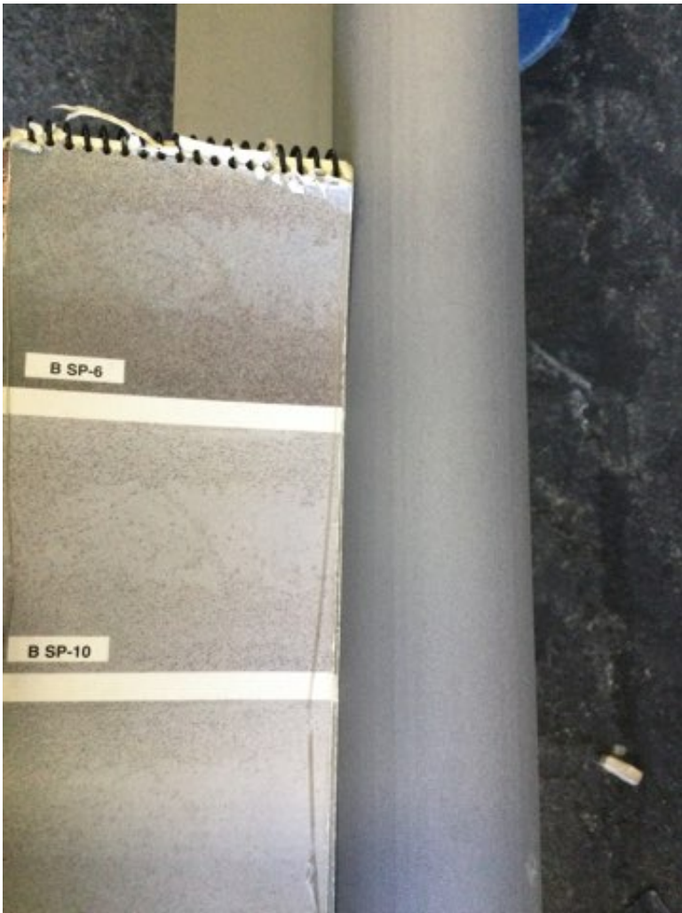
Photo Description: Grit blasted Surface visual comparison to SSPC -VIS 1 guide SP10 cleaning
