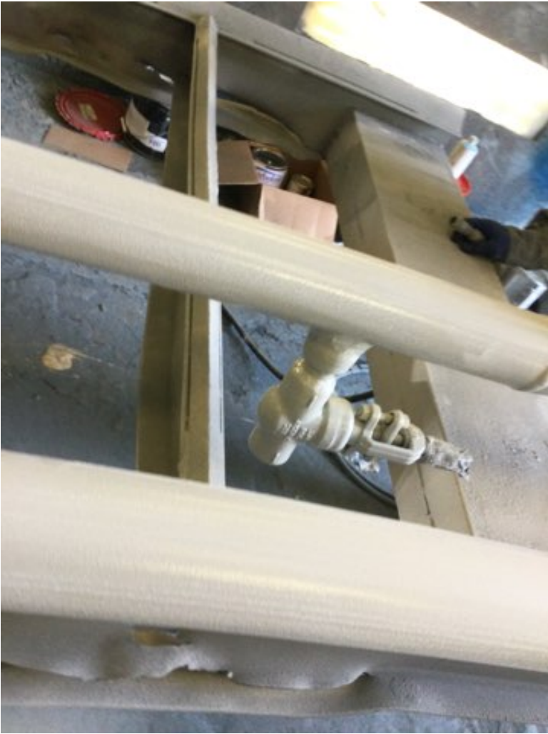
Photo Description: Epoxy coated
